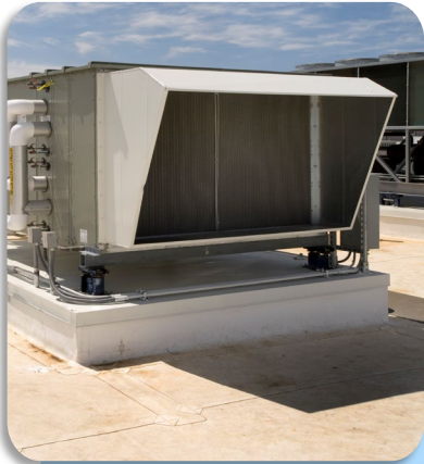
Commercial Rooftop Units
