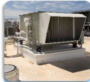
Commercial Rooftop Units
