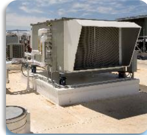
Commercial Rooftop Units
