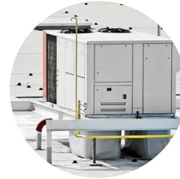
Commercial Rooftop Units
